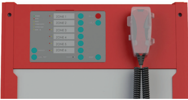
Control/Indications & Firemen microphone at access level 2
